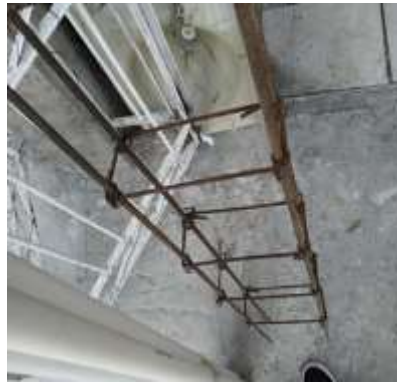
Figure 2. Column with a dimension smaller than that provided by NBR 6118 (ABNT, 2018).
