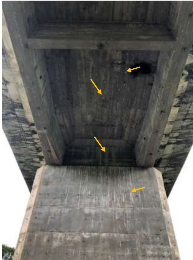
Figure 8. Efflorescence incidence spots.
