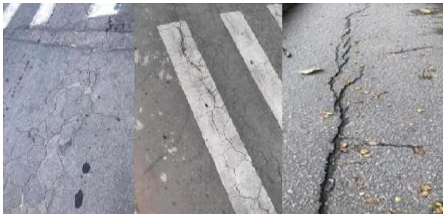
Figure 4. Longitudinal crack found in the central region of the city
