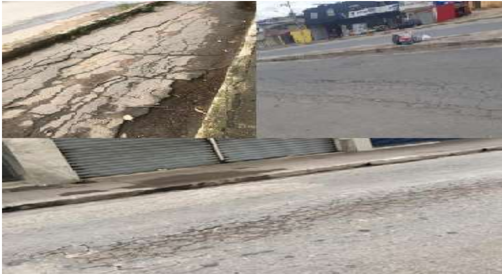
Figure 5. Interlocking cracks without preferential directions
