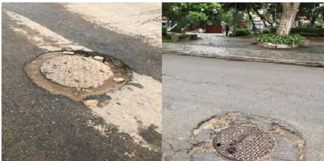
Figure 6. Pans or holes identified
