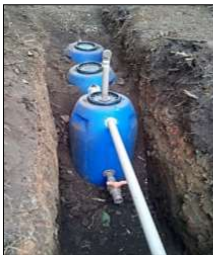
Figure 2 - EST after installation in Botucatu/SP.
