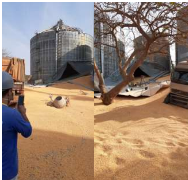
Figure 5. Debris from the silo that broke in MT.
