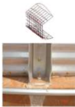
Figure 7. Deformation of the column due to local instability.
