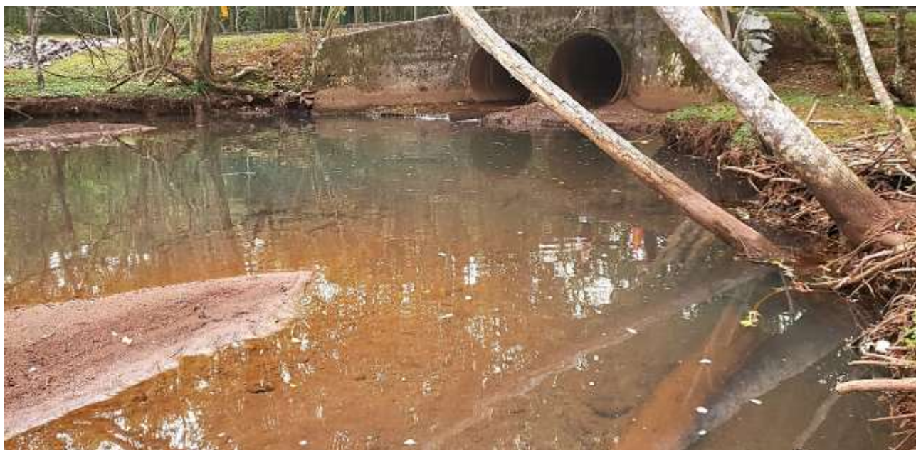
Figure 7. Sediment Accumulation inside a double-tube concrete culvert located near the Municipal Lake.
