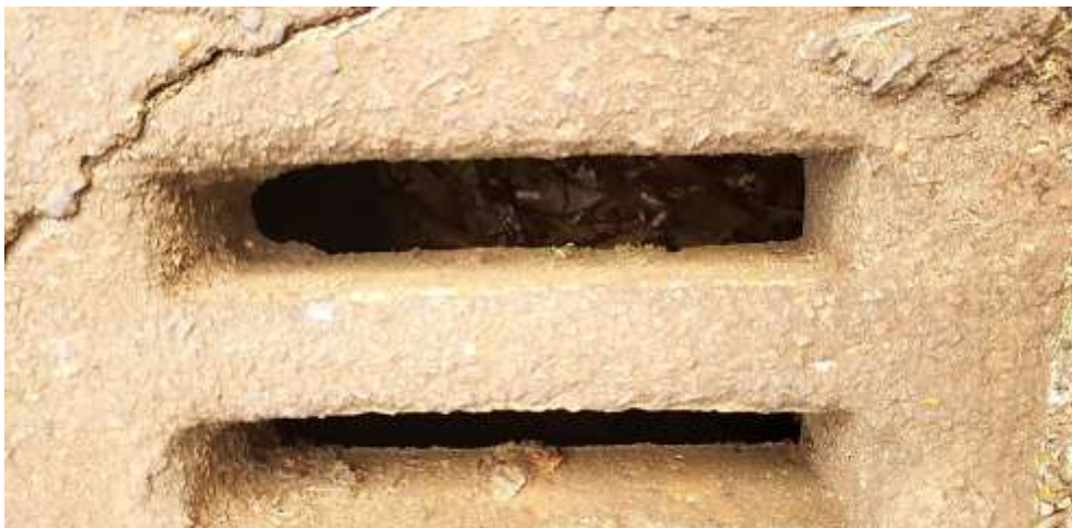
Figure 6. Leaf accumulation inside a drain, located on the Municipal Lake vicinity.
