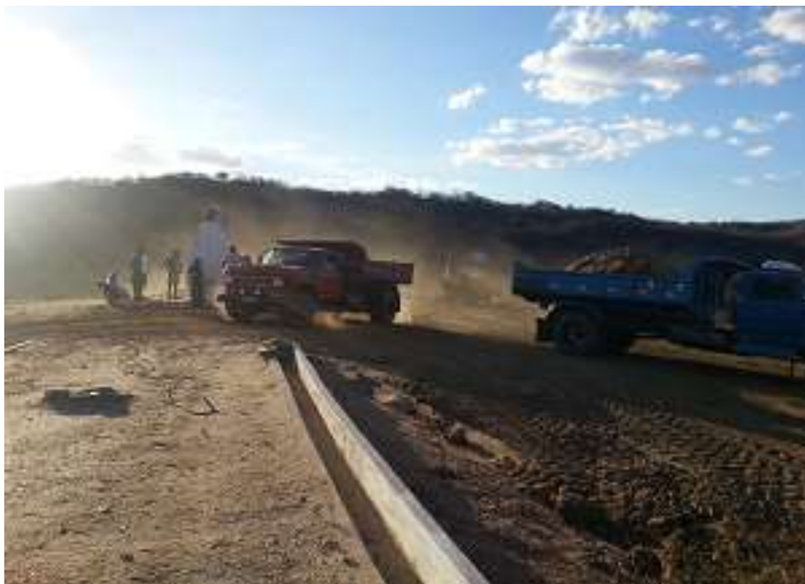
Figure 4: Bucket trucks transporting material and depositing it on the wall opposite the weir, strengthening it for a possible increase in its capacity.
