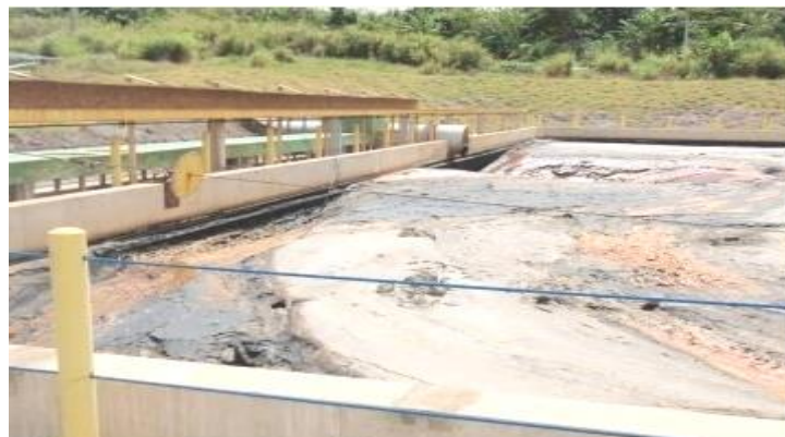
Figure 7 – Solids accumulation in the tank.(Source: the author)
