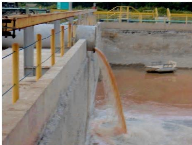
Figure 2- Inlet pipe feeding the tank (source: Dow Química do Brasil )
