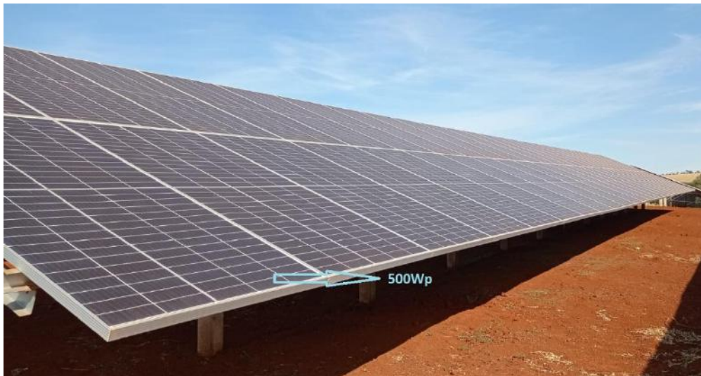
Figure 2. Fixed photovoltaic system installed in Cascavel, Paraná.
