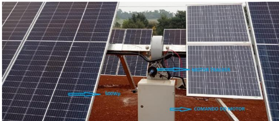
Figure 1. Tracker photovoltaic system installed in Cascavel, Paraná.
