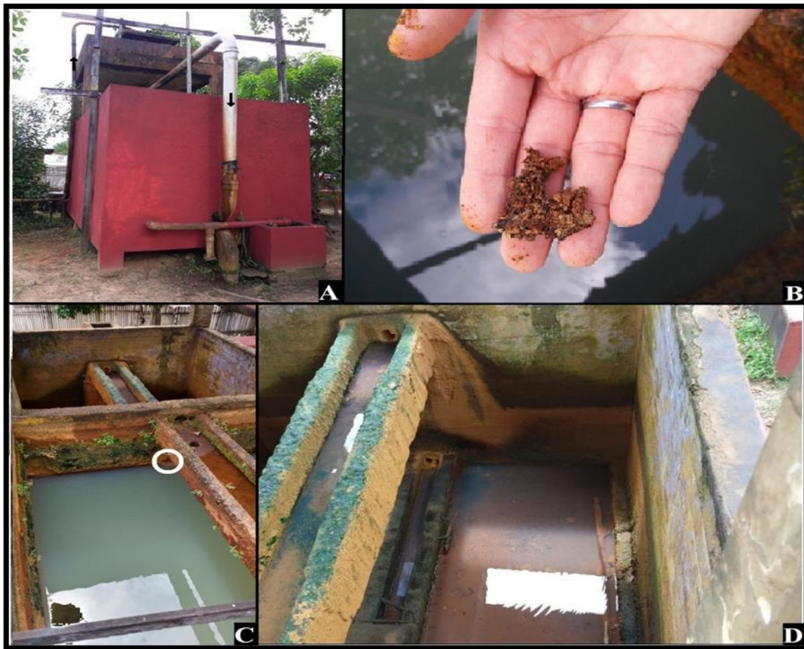
Figure 5 - (A) Aerator and filter (arrows showing the water path); B: Sediment from the filter wall; C: Compartment 1 (circle showing “shortcut”) and 2 of the filter; D: Filter compartment 2.
